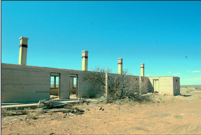
AT&SF Section Houses were built by the railroad to house the track crews maintaining the railroad. Located on the Armendaris Ranch at the "Lava Siding." There are very few Section Houses still standing in New Mexico.
